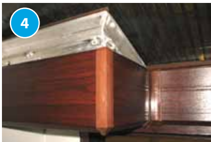
Raised Leg Box Gutter: Fit all of the internal side clads as standard.
