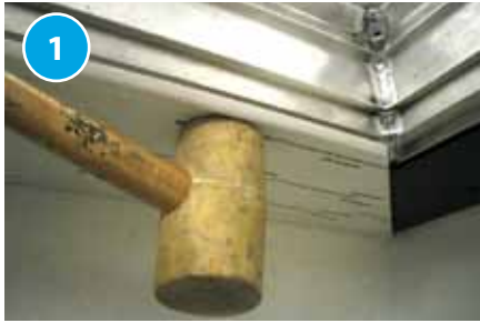
Box Gutter: Position then knock the box gutter under clad in to position using a rubber mallet.
