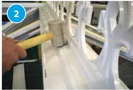
2 Starting at one end knock the top cap in to position using a rubber mallet.
